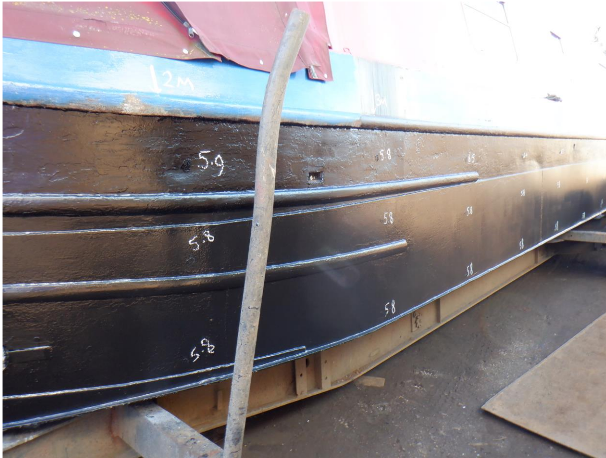
Fig. 1 - Diagram showing ultrasound thickness readings on the flat-bottomed hull, tuck/swim and port and starboard sides of SXXXXXX. Plan and side views. All readings were mapped in millimetres.
